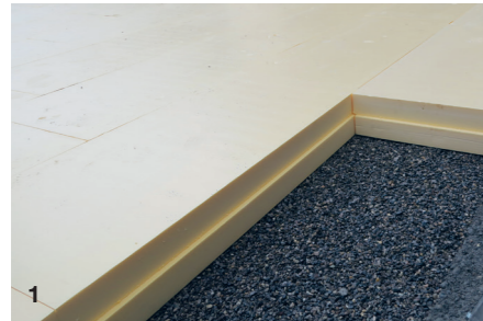
1 Insulation boards with a thickness of 160 mm are laid on a layer of chippings.
