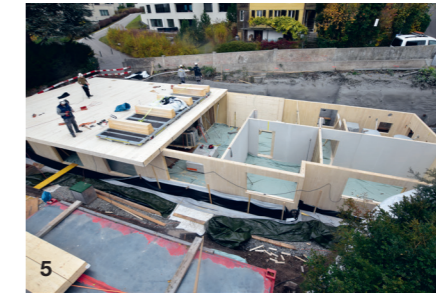
5 The cross-laminated timber panel above the basement acts as a floor slab.
